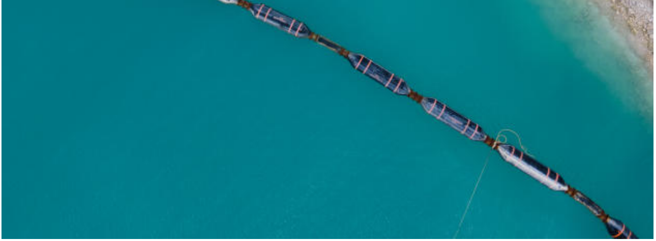
The sand is pumped from the bottom of the ocean and then transported to land through large pipes on Felivaru Island (Maldives) in February 2022. MATHIAS DEPARDON FOR "LE MONDE"
